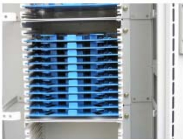
144 FO Splicing Unit
