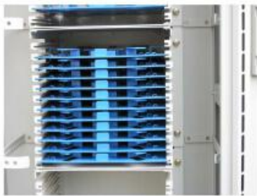
144 FO Splicing Unit
